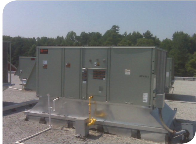
New rooftop air conditioners are helping Clayton County taxpayers save significant energy while improving comfort and employee productivity.
